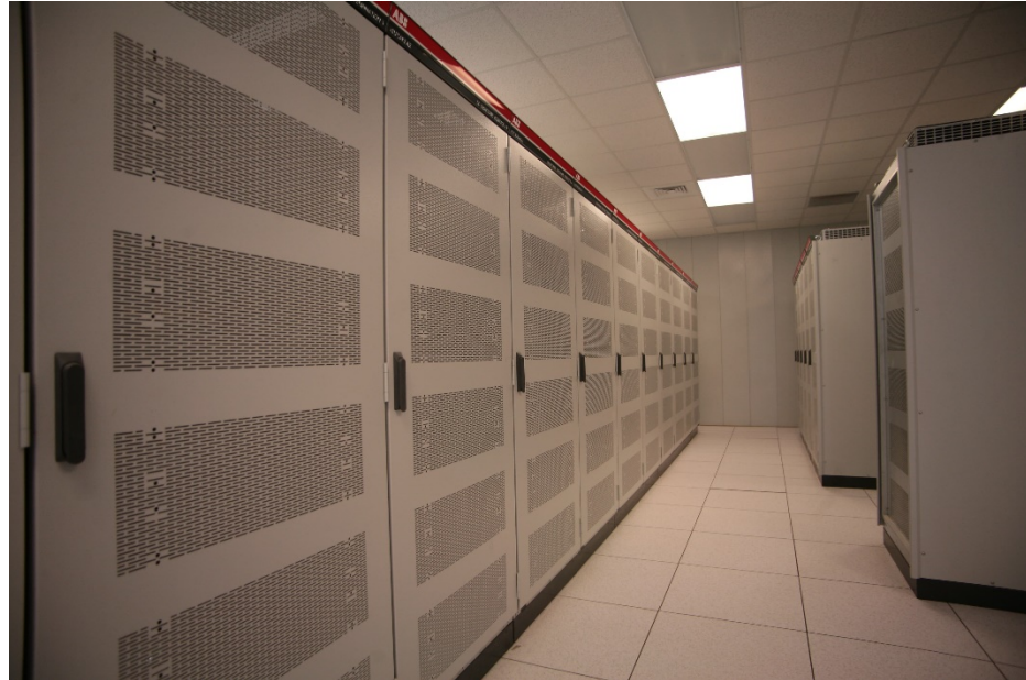
Plate 5.24 – Typical Control and Protection Cubicles Image: ©ABB
