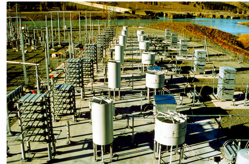
Plate 5.11 – Typical AC Switchyard Harmonic Filters Image: ©ABB
