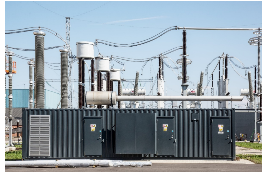
Plate 5.13 – Typical Diesel Generator Image: ©ABB
