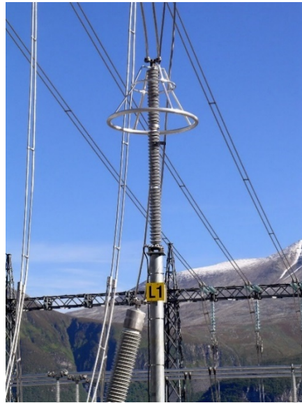
Plate 5.7 – Typical HV Surge Arresters Image: ©ABB
