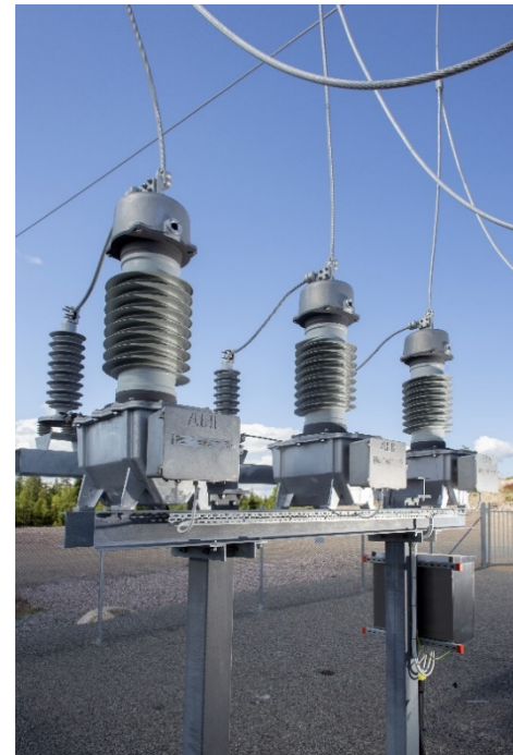
Plate 5.16 - Typical Voltage Transformer Image: ©ABB
