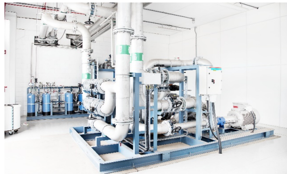
Plate 5.22 – Typical Water Pumping Station Image: ©ABB
