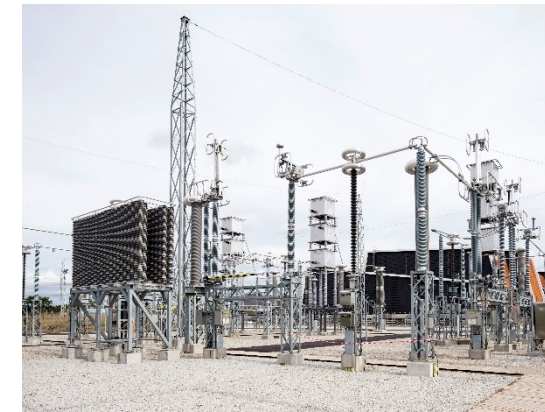
Plate 5.8 – Typical Lightning Masts Image: ©GE
