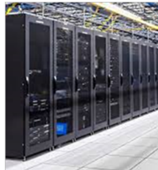
Plate 5.38 – Typical cabinets configuration (Copyright – B&M FOC Review Report Issue D Sept. 2018)
